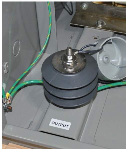
Figure 6: Output Surge Arrestor without cap
