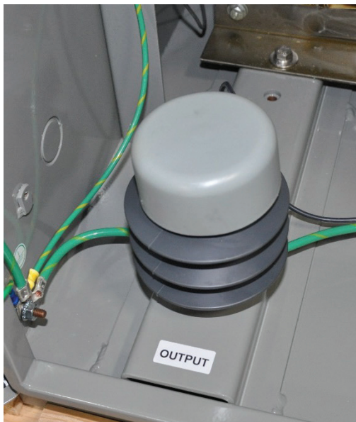
Figure 5: Output Surge Arrestor with cap
