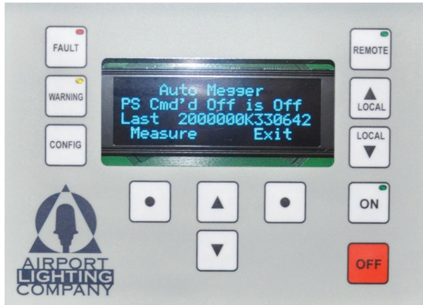
Figure 15: The Megger Screen
